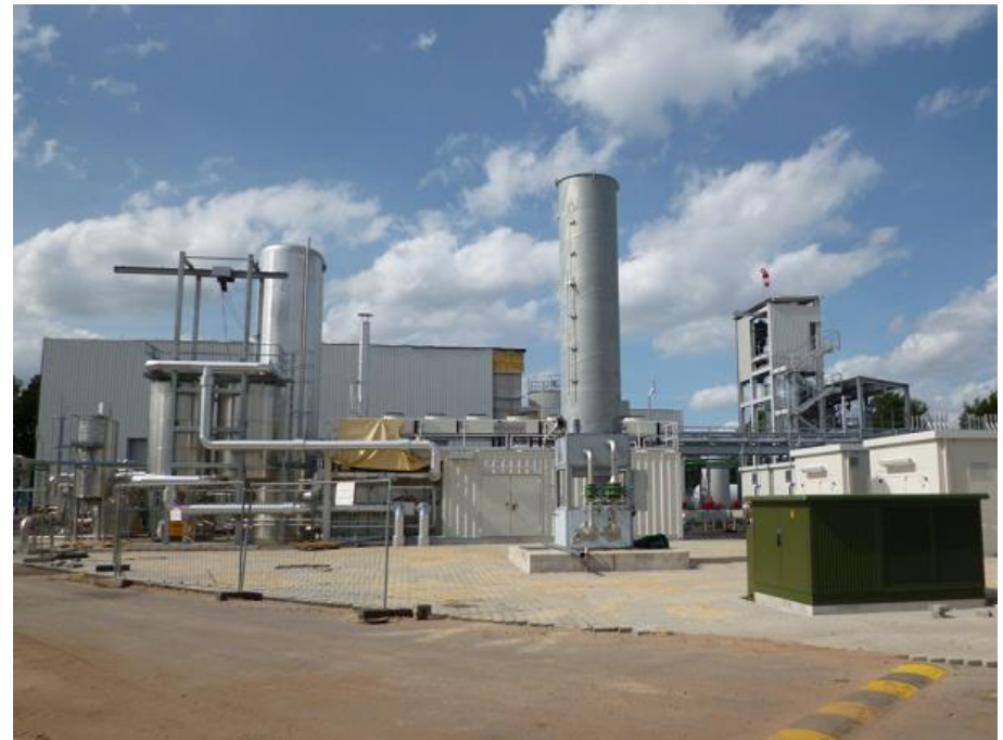
Minimum Viable Product: 6.2MW Werlte Pilot Plant, commissioned June 2013
