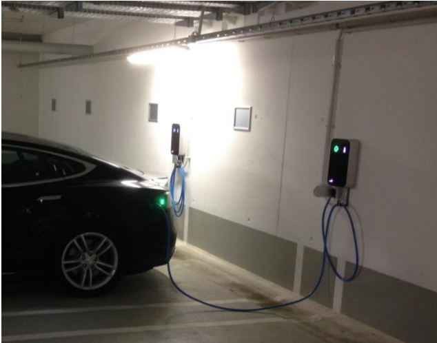
Charging solutions for company car fleets
